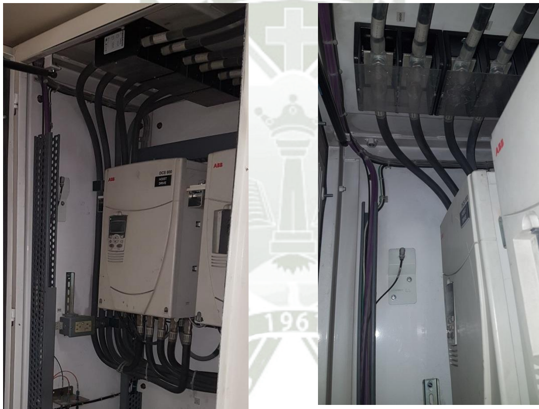
Figura 4-11: Sensor de ArcFlash Gabinete 520VAC
