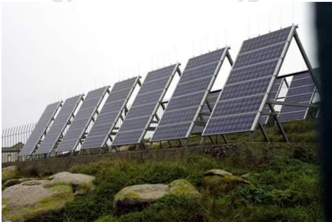
Fig. [26]. Paneles solares
