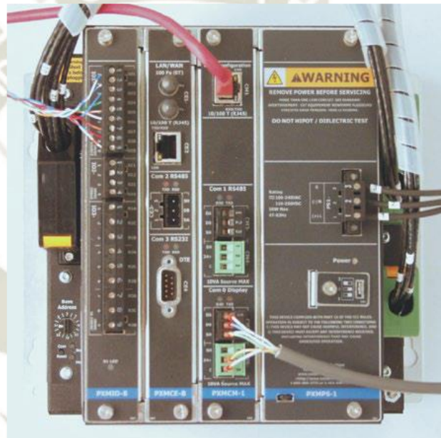
Figura 3-5: Eaton Power Xpert Meter 8000 [59].
