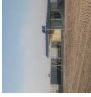
03 43 kWp Solar powered water pumping and desalination system (43kWp in Dubai, UAE)
