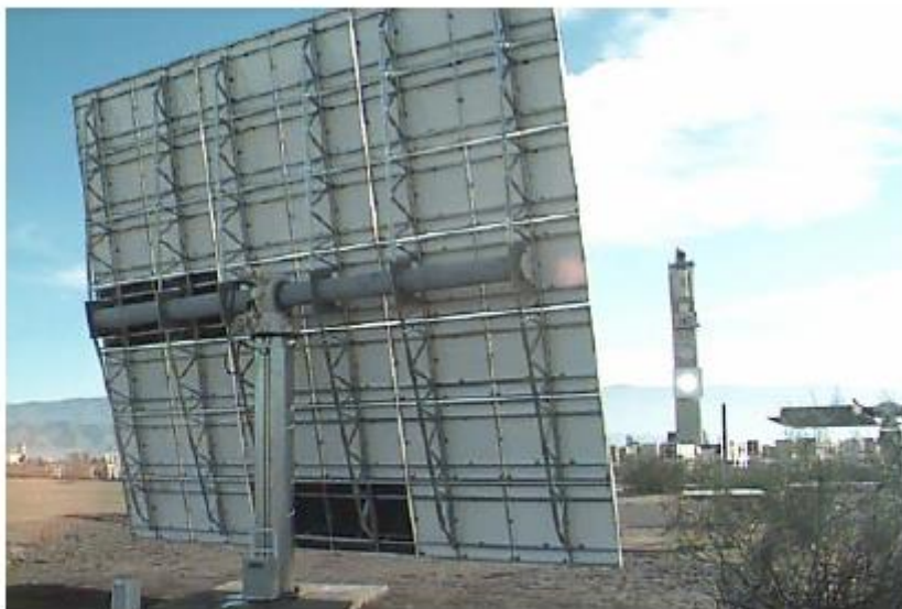
Figure 4. Back structure of the Colon 70 heliostat with image shown on tower.
