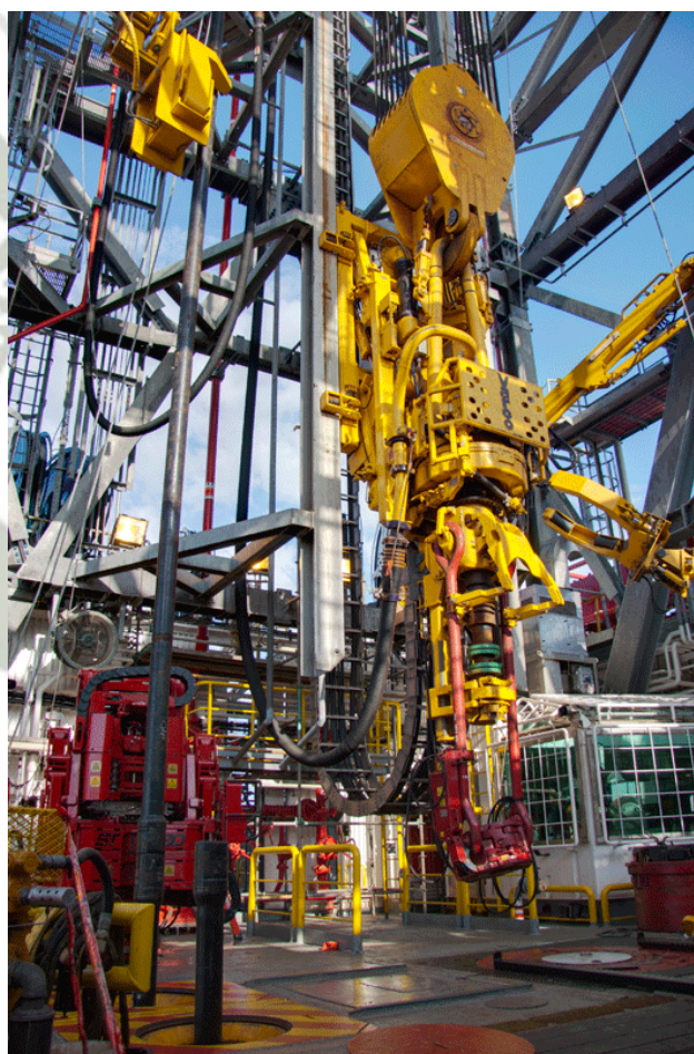
Fig. 3.11 Top drive TDS9 Varco.
