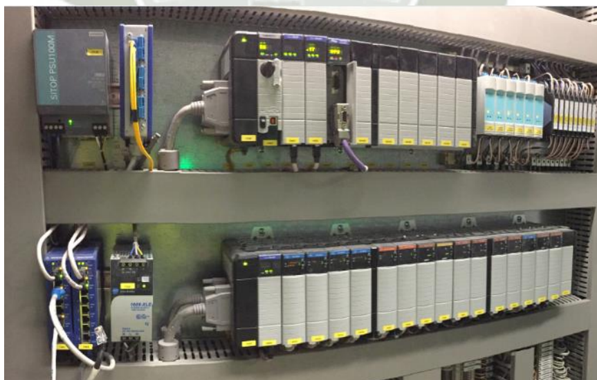
Figura 6.4.b Tablero de control principal
