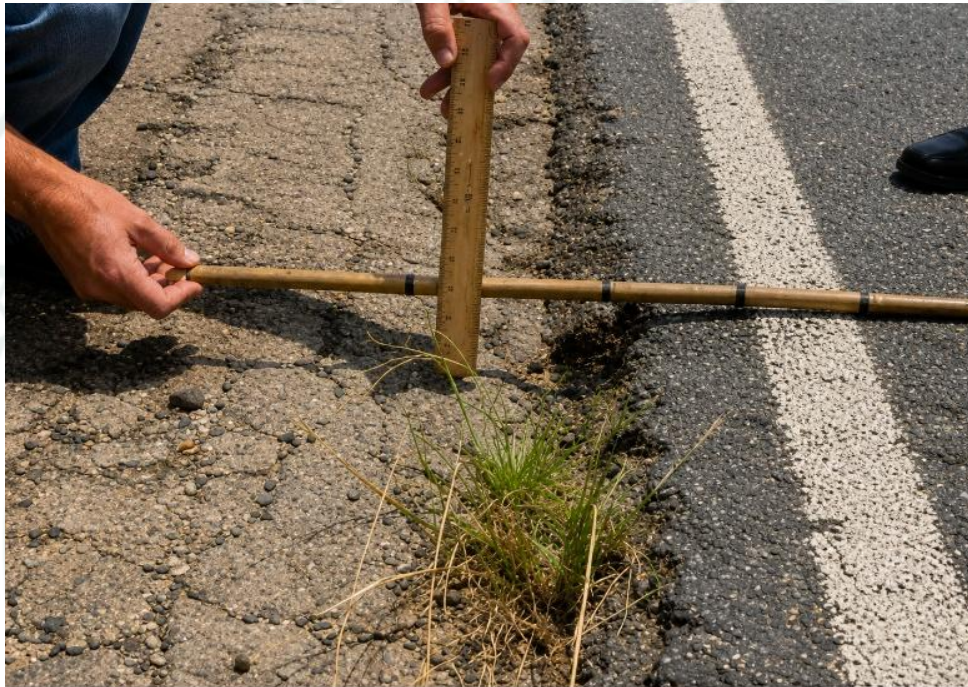
FIG. X1.26 Medium-Severity Lane/Shoulder Drop-Off
