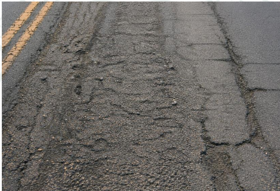
FIG. X1.52 Medium-Severity Weathering and Raveling
