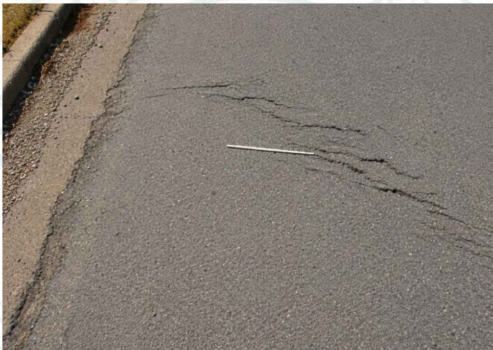
FIG. X1.48 Medium-Severity Slippage Cracking
