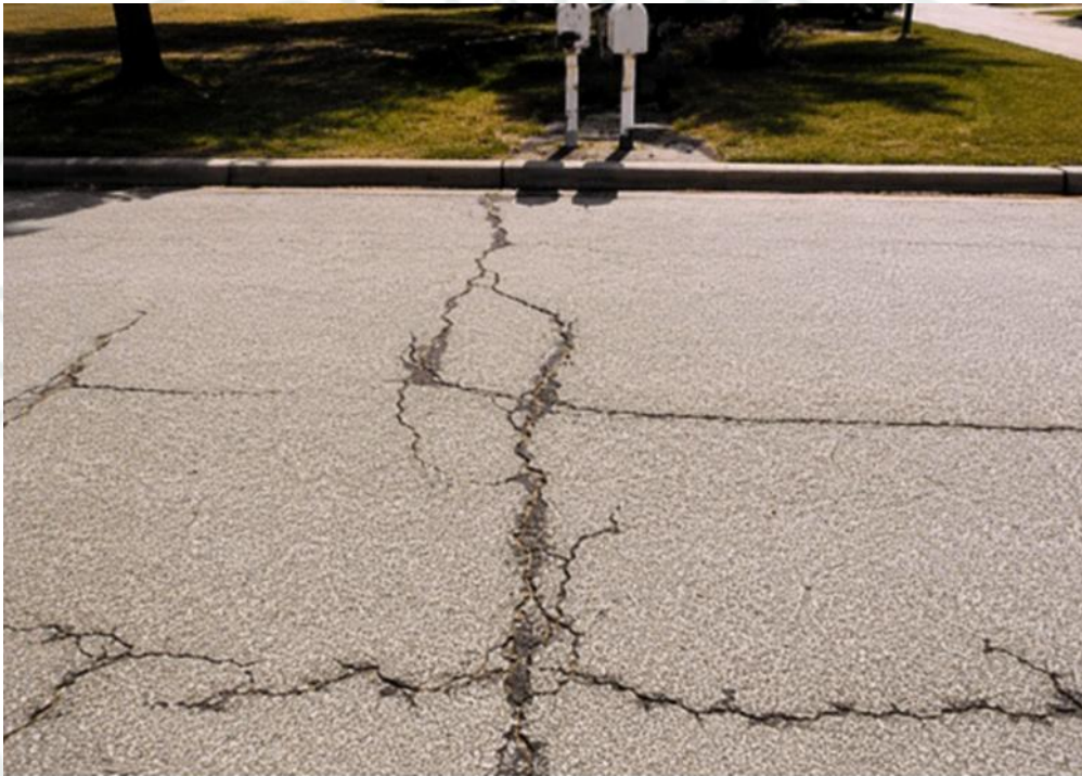
FIG. X1.8 Medium-Severity Block Cracking
