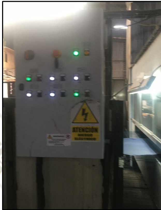
Figura 27: Tableros de control
