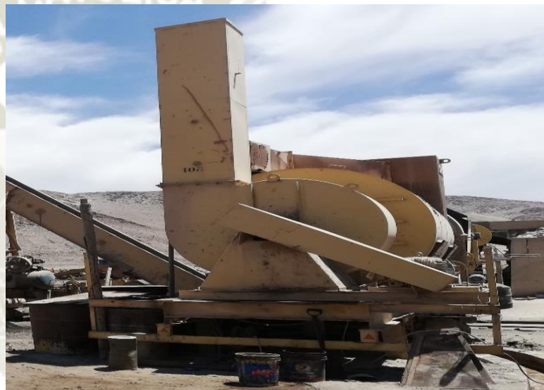
Figura 11. Exhaustor de Gases
