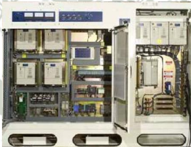
Fig. 6.16 Gabinete de control
